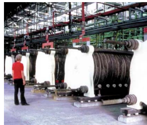
Older Norsk Hydro Hydrogen Plant
